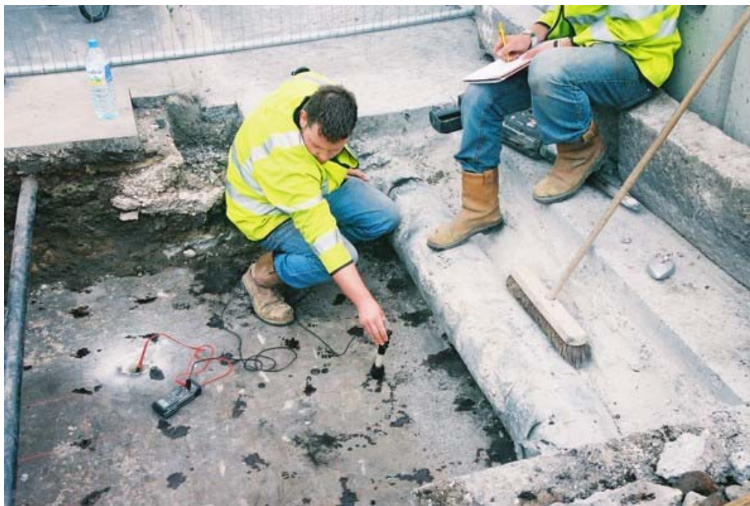
Figure 2.1: Preliminary measurements in a preview study on the crown of an arch highway structure (from SAMARIS Report D21)
